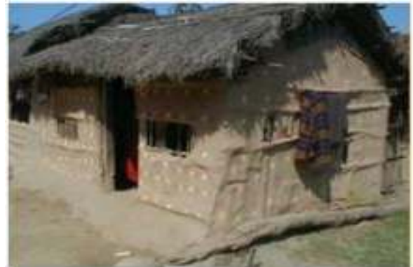
Figure 4 Shading device and small window detail from a kacha house in Rajasthan
